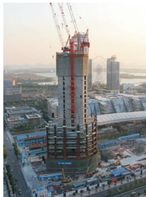
The control system for the Die Climbing Machine , which used to build the Suzhou international financial Center, which is the tallest building in Suzhou, is designed by our company .
