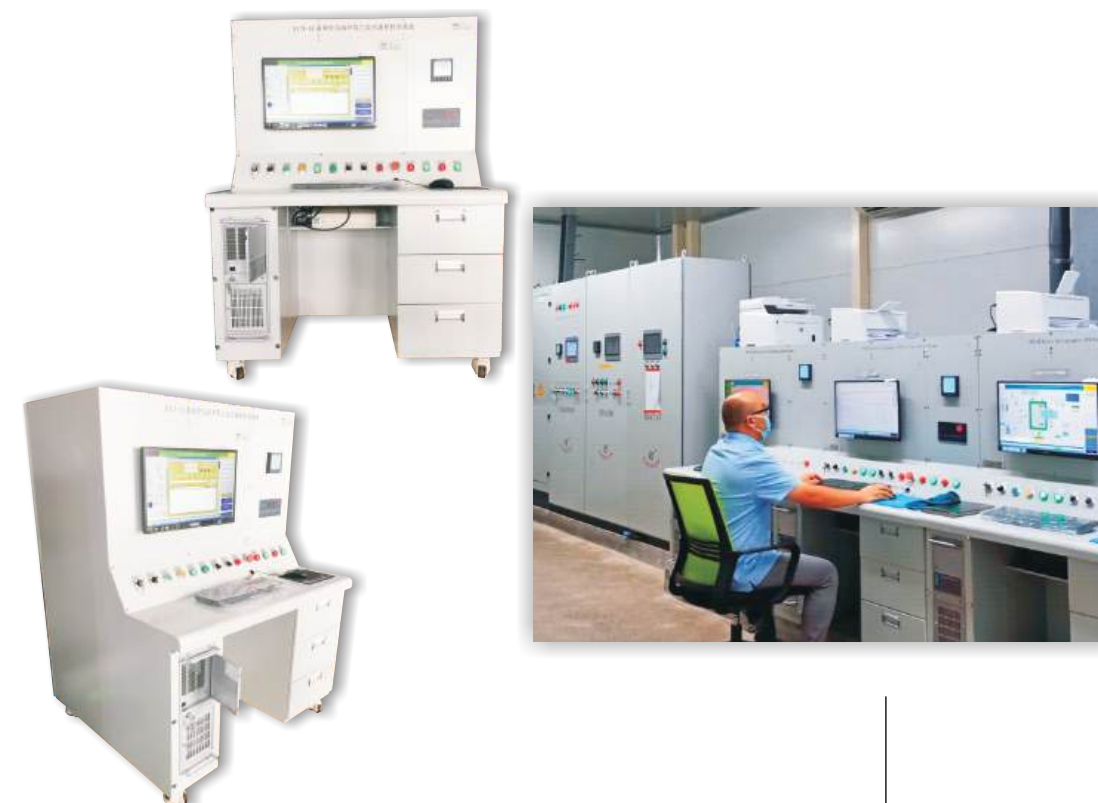
Integrated Control System
